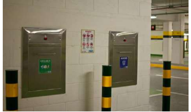
Load Station – Provided on every floor; mixed and recyclable waste.
