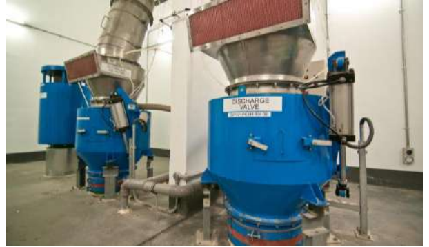
Discharge valve – Automated operations and controlled waste release.
